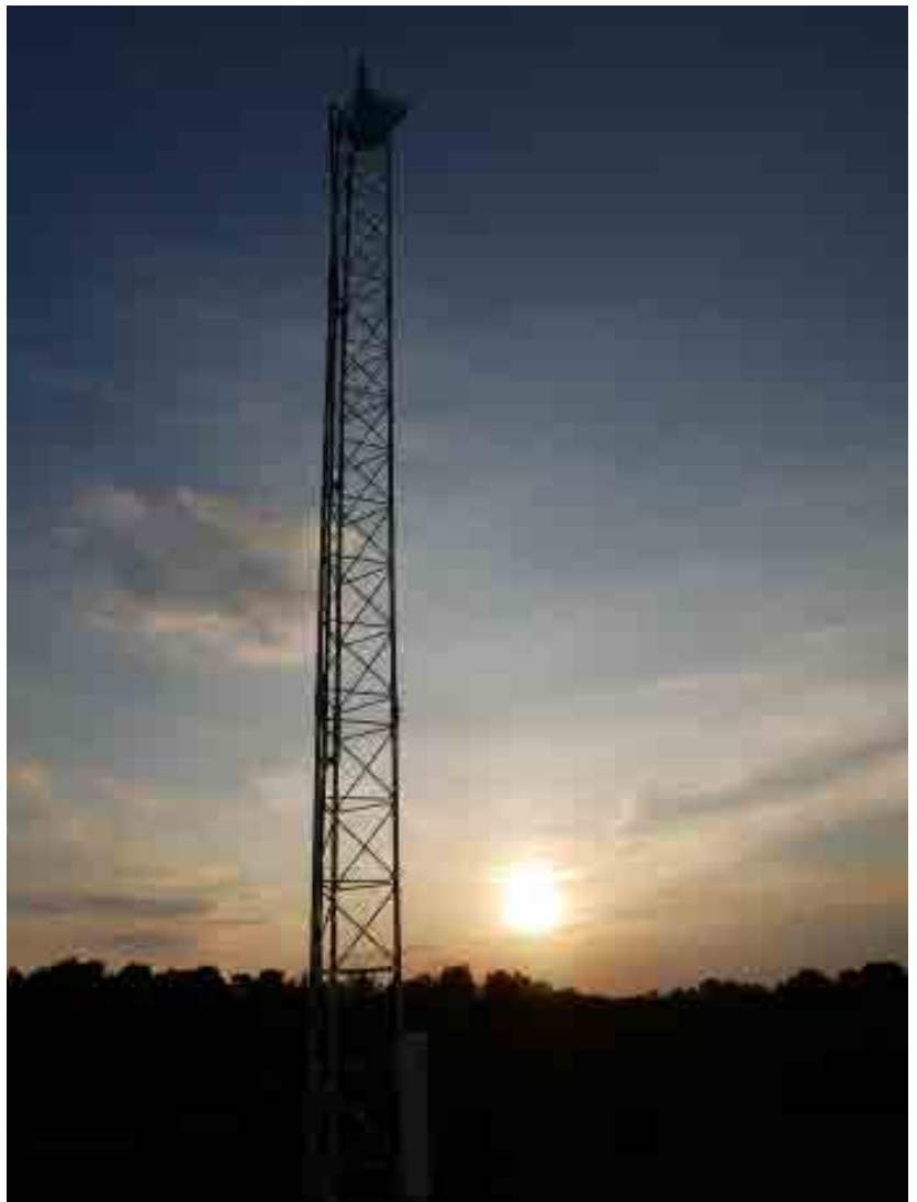
Pictured above is an 85ft Rohn 45G Tower and gamma nu 20dBi Gain RF Cascade Link Donor Antenna serving one of four 20W ICS 1900MHz Band 2 LTE Cellular Repeaters Providing Exterior Cellular Voice, Text, Data, & IoT Coverage to over 250 acres at one of the world's largest food processing and distribution facilities. A Panel Antenna on this tower also serves as an RF Cascade Wireless Link relaying T-Mobile-Sprint signal to the facility's In-Building CEL-FI QUATRA 2000 Active DAS Hybrid.
